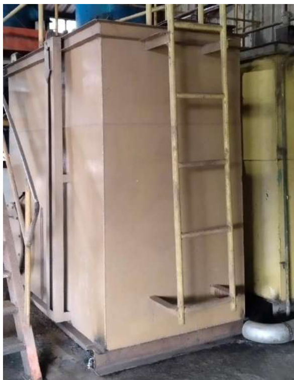
Gambar 21. Storage Tank PKO Sementara
